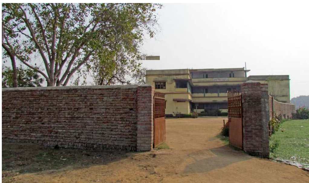
New boundary wall for the expanded school grounds and new gate with vehicle access
